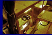
A 100w solar charger would be used to charge the 2 12V batteries hidden behind the power panel.
